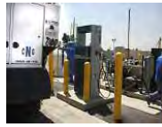
GESI installation for Rancho Cucamonga
